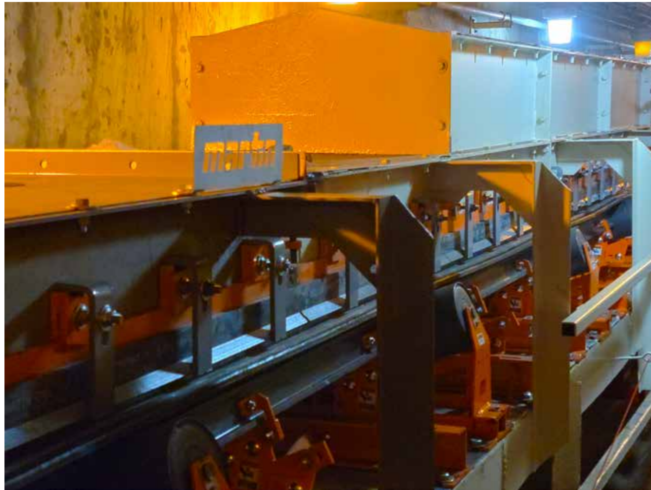
A well-designed loading, settling and stalling zone require safe components that protect the belt and the surrounding work environment.
