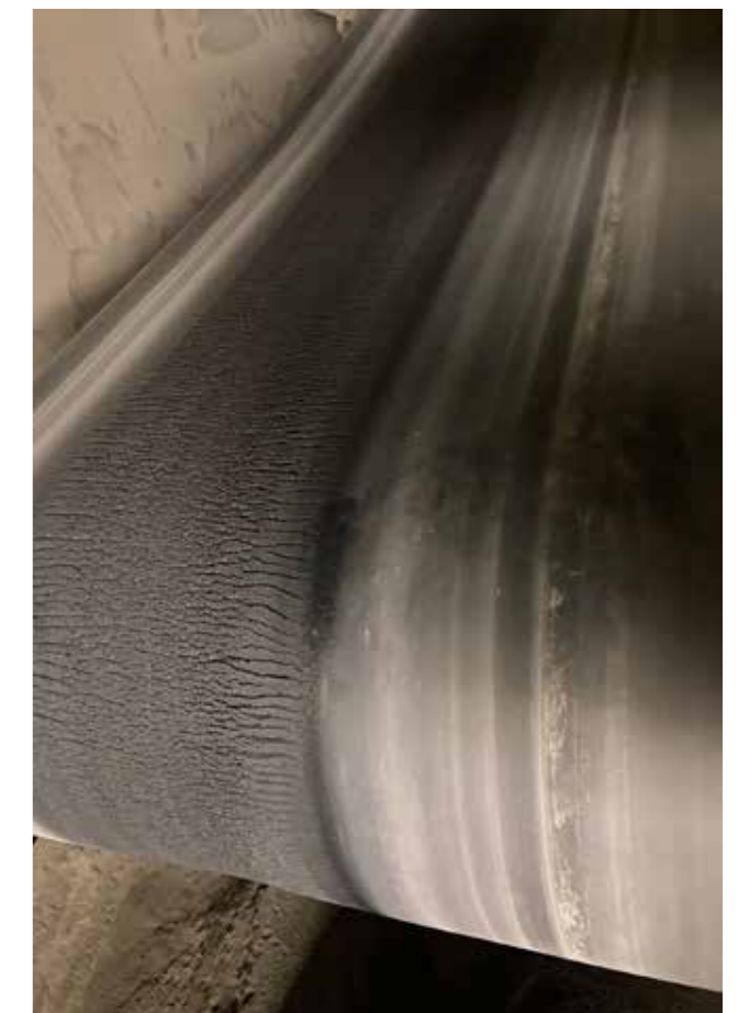
Cracking up. Without ozone and UV resistant covers, wear and tear is accelerated.
