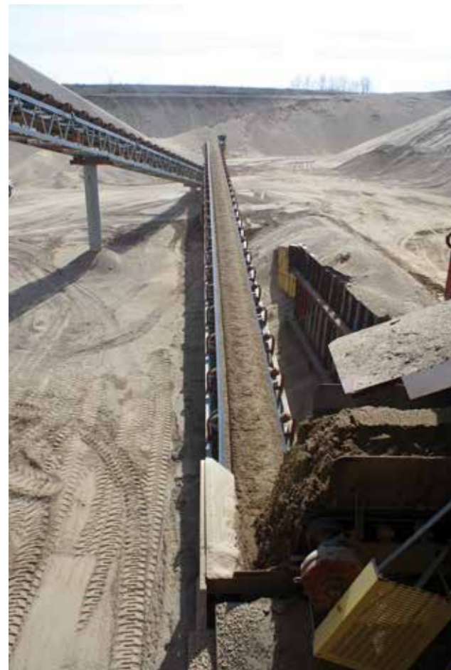
Changes in belt speeds or material properties can drastically impact the efficiency of a non-linear transfer point.
