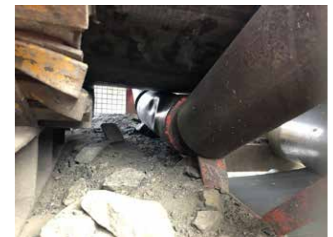
Unclean environments and damaged rollers can accelerate wear.
