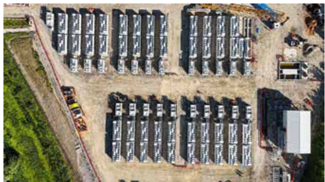
The BESS at Ferrybridge C will have a capacity of 150 megawatts - enough to power 250,000 homes (Credit: Getty Images)
