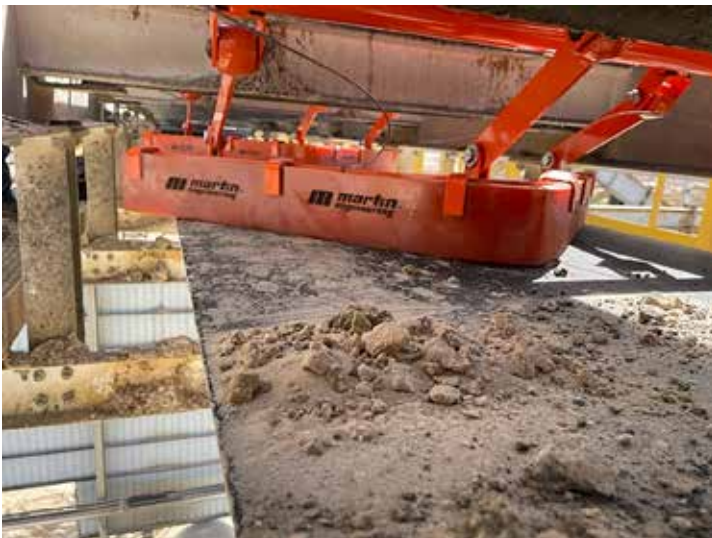
Figure 5: The workhorse of tail pulley protection, the V-plow safely clears debris without harming the belt.
