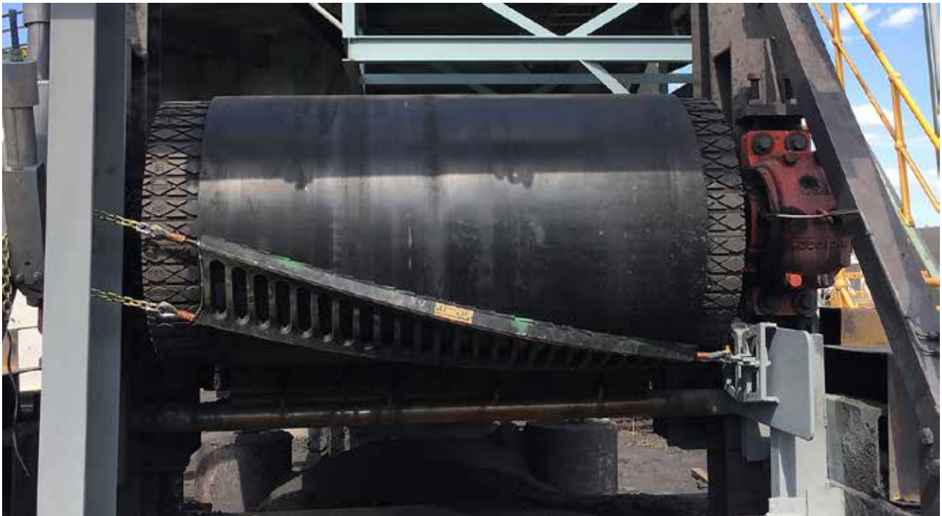
Figure 1: Innovative belt cleaning technology can improve cleaning, safety, and the cost of operation.
