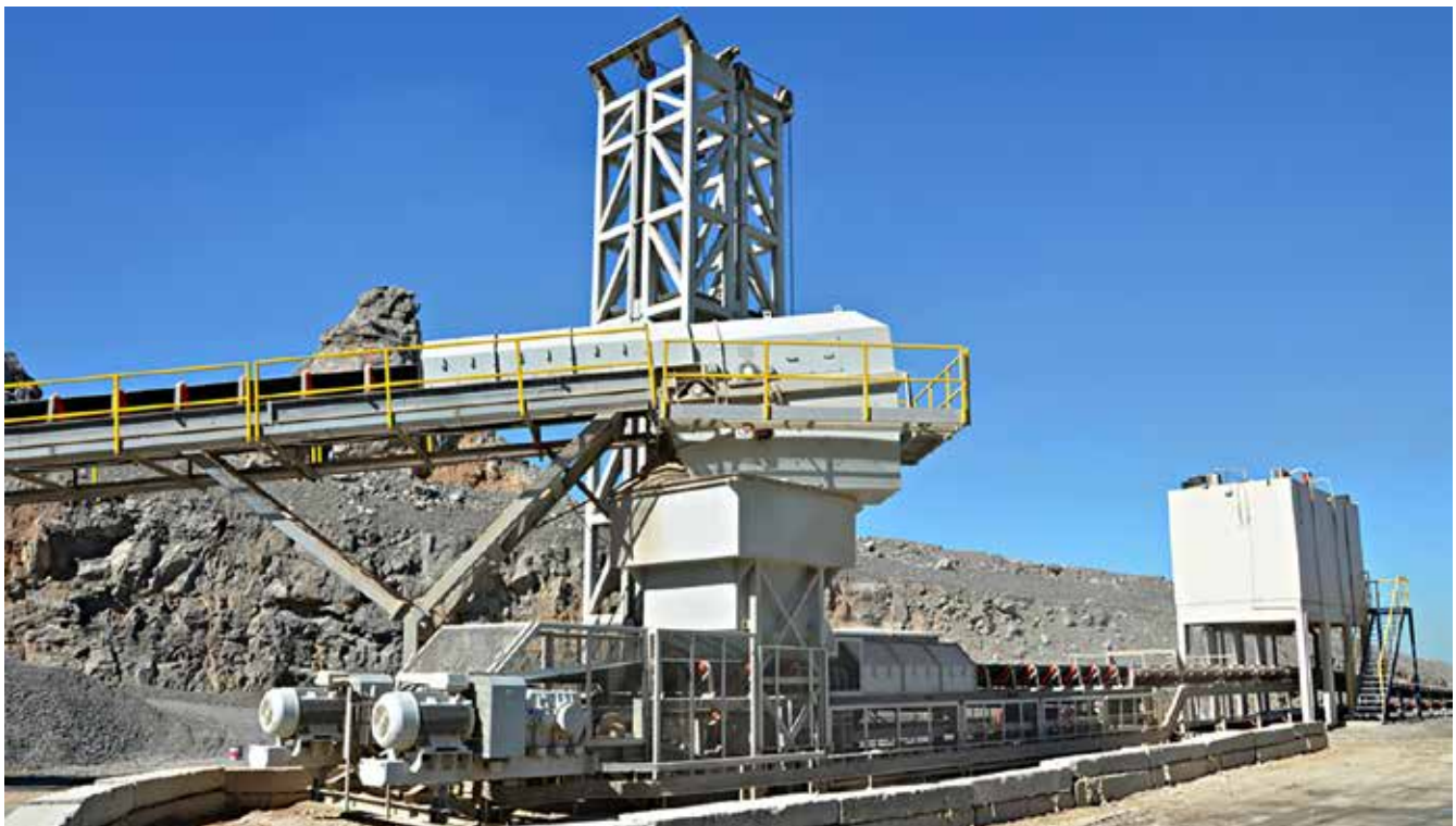
Conveyor systems – Quarry Mining
