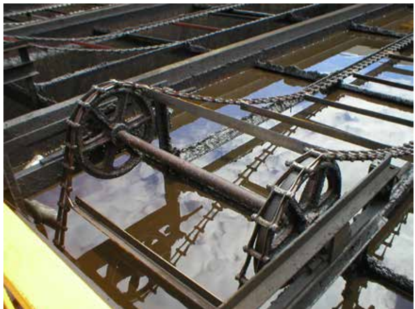
Cobalt chains clarifier tank
