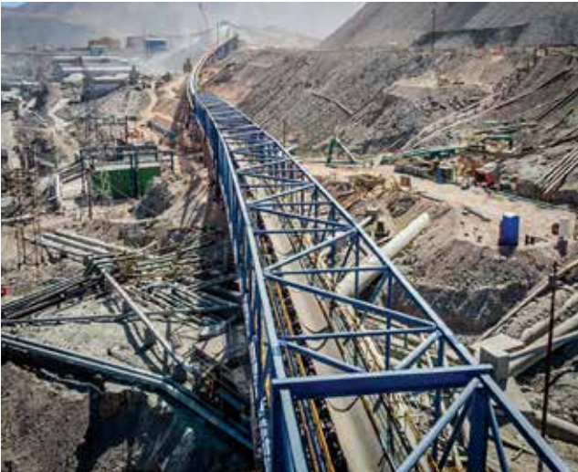
Overhead mining conveyors
