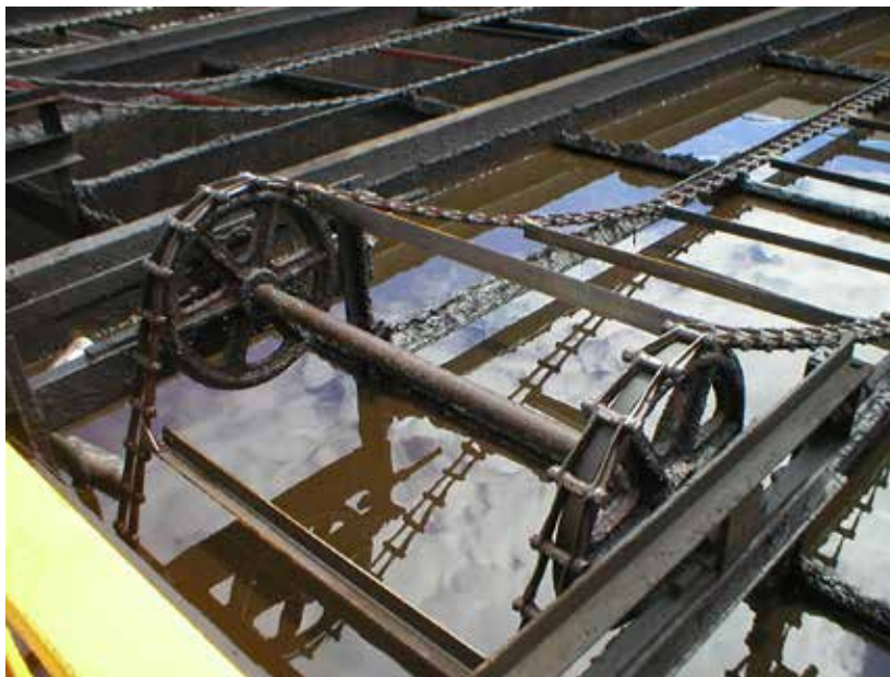
Cobalt chains clarifier tank
