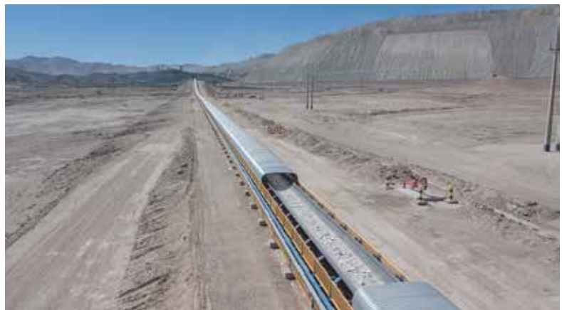
First ore on the TAKRAF Overland Conveyor with gearless drives at Chuquicamata, Chile.
