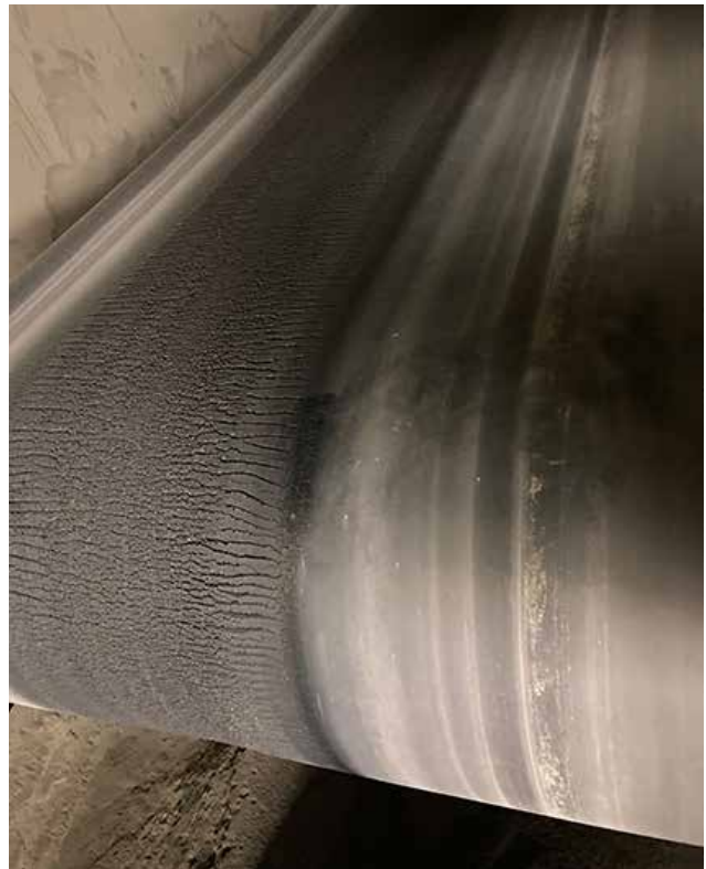
Cracks deepen under the repeated stress of passing over the pulleys and drums.
