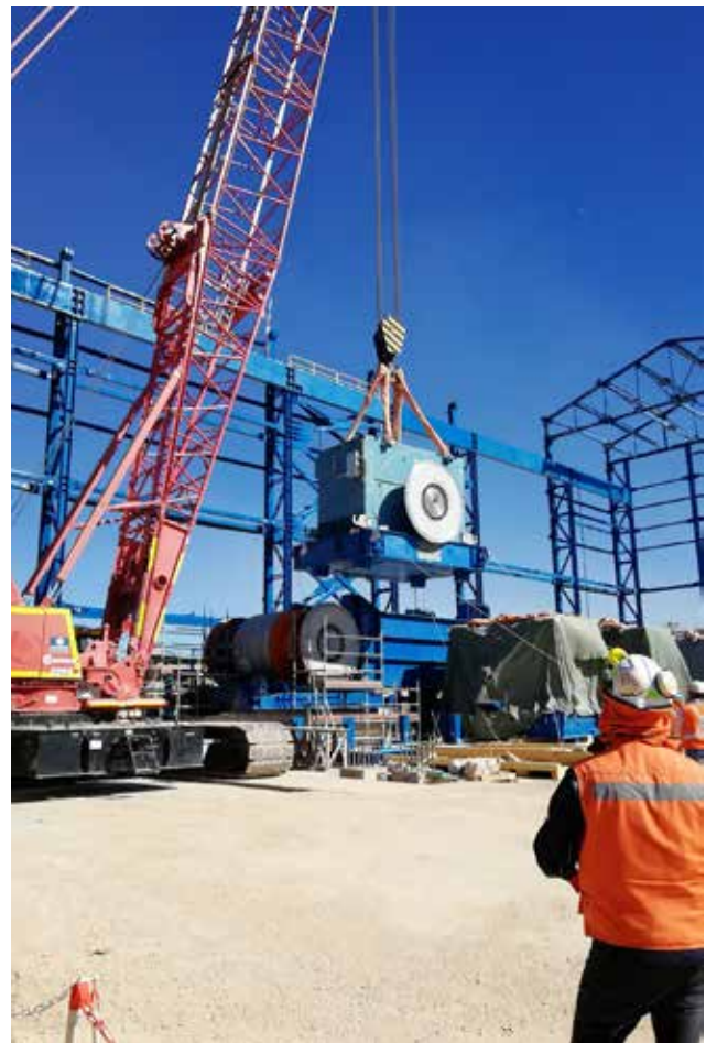
The entire drive arrangement, including stator, rotor, bearings and frame, arrived at the Chuquicamata site assembled and tested as a single, ready-to-install unit.
